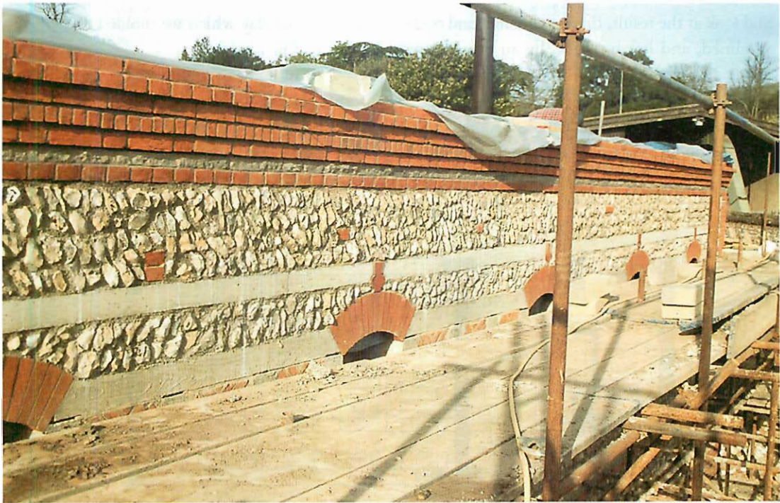
Here we see the handling of brick, headers, flint, and stone, that we worked out, course by course, to give the cornice at the top of the north wall a true I-like character. It took many experiments, and every course had to be placed by eye, in mock-ups, to make the whole thing come out right.
