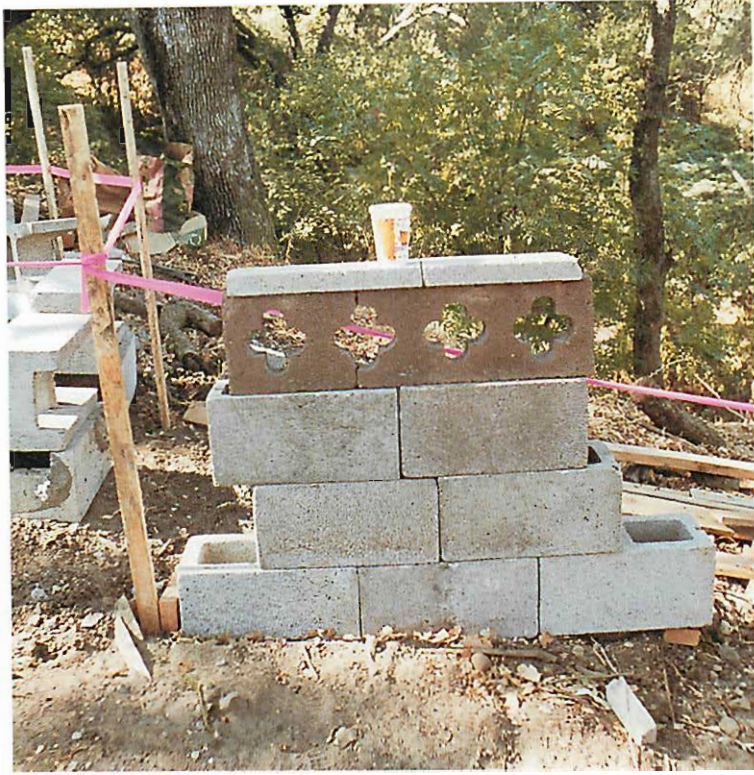
The work of finding beings always starts at the very simplest level, as we see in our efforts to make rosettes in concrete during a construction experiment from one of our building sites.
